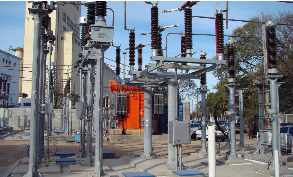
Santa Fe Port transformer station
